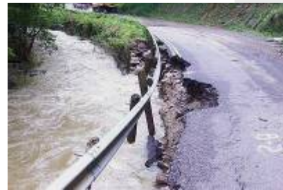
Severe road damage and washout
