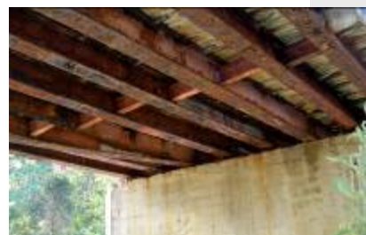
Rusted beams under wood deck
