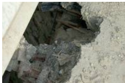
Deterioration of asphalt and exterior beam
