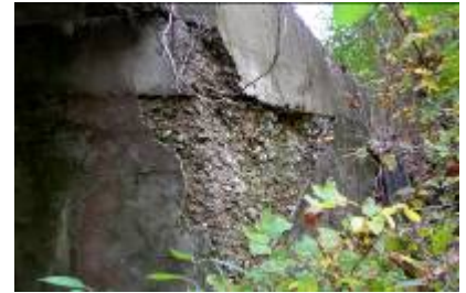
Deterioration of bridge wall
