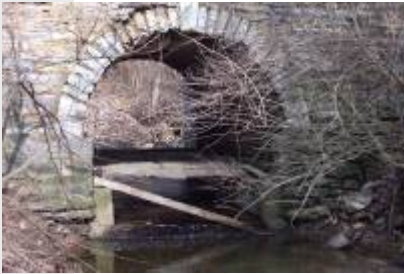
The old bridge in need of replacement
