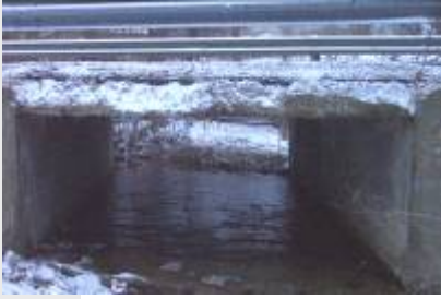
Bridge to be replaced on Crossley Road
