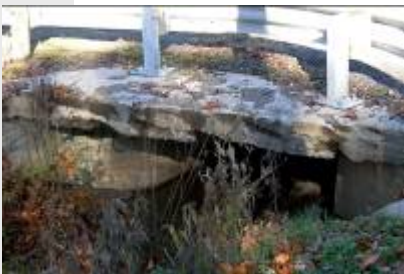
Concrete wear on old bridge
