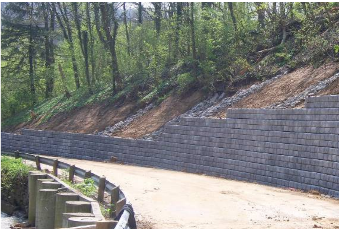
The new Redi Rock Wall along side of road and new H-Pile Wall along creek
